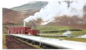
Figure 3.7 A geothermal generating station transforms thermal energy to kinetic energy to electrical energy.
